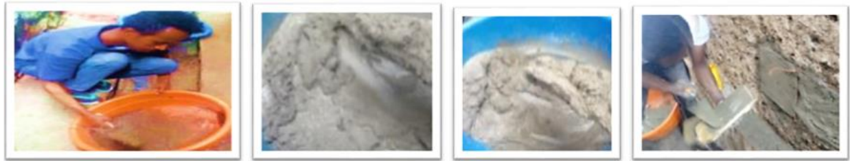
Figure 14 Process of making plaster on the wall surface, for third coat plastering
